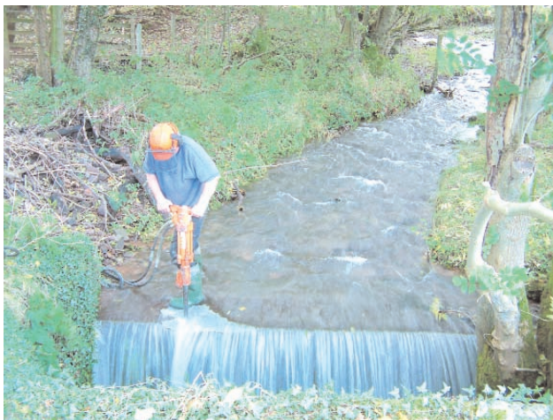
Fig 4. A redundant weir on a trout stream in the Rhiangoll system
