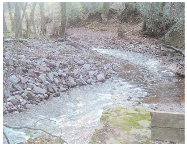
Figure 2 - Directly after removal. Note the pipe preserving the flow down the leet)
